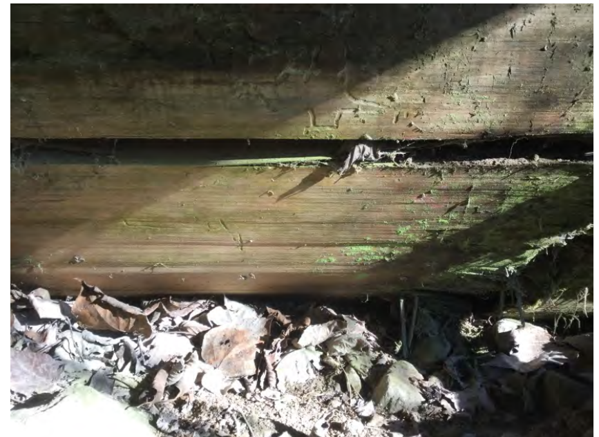
Horizontal crack on left bank log sill; full visible length 30mm gap
