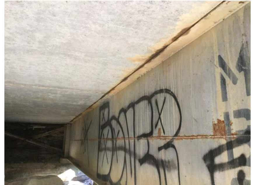
Indication of water leaking through deck joints and grout pockets
