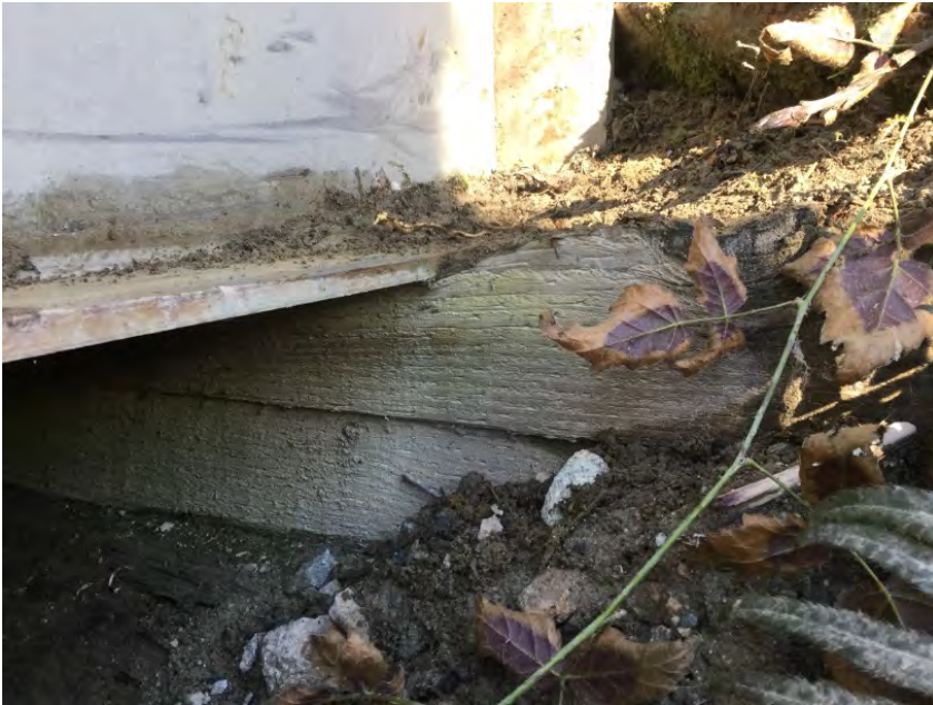
Timber shims on left abutment rotting and indications of crush, downstream shim shown here
