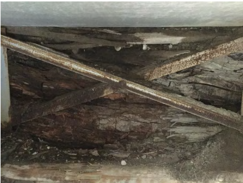
Ballast wall condition, left bank
