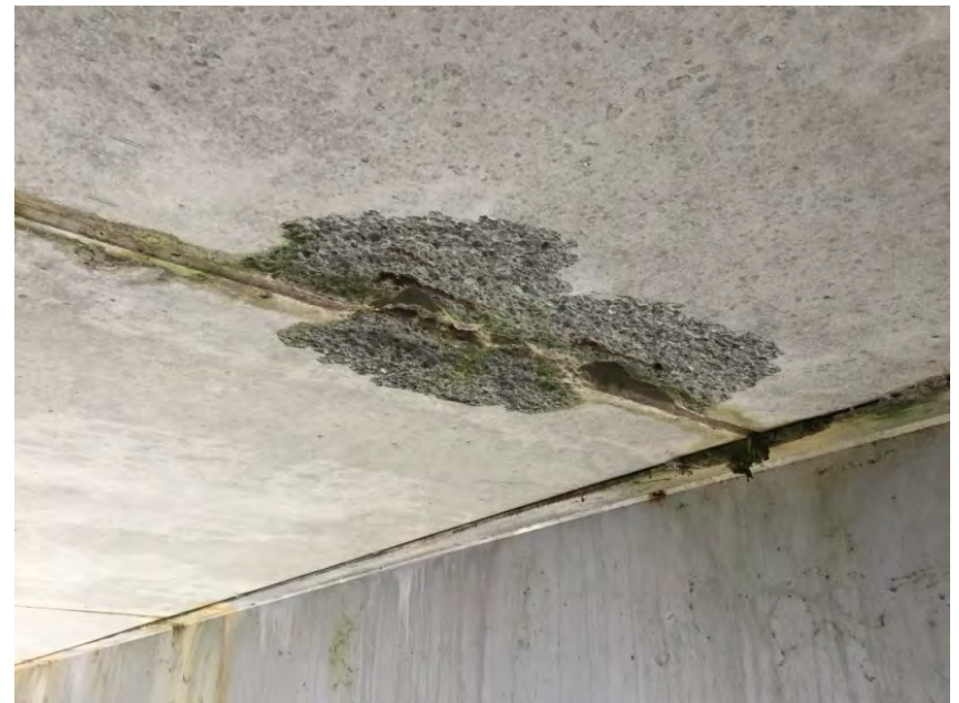
Damage noted to panels 1 and 2 on right approach
